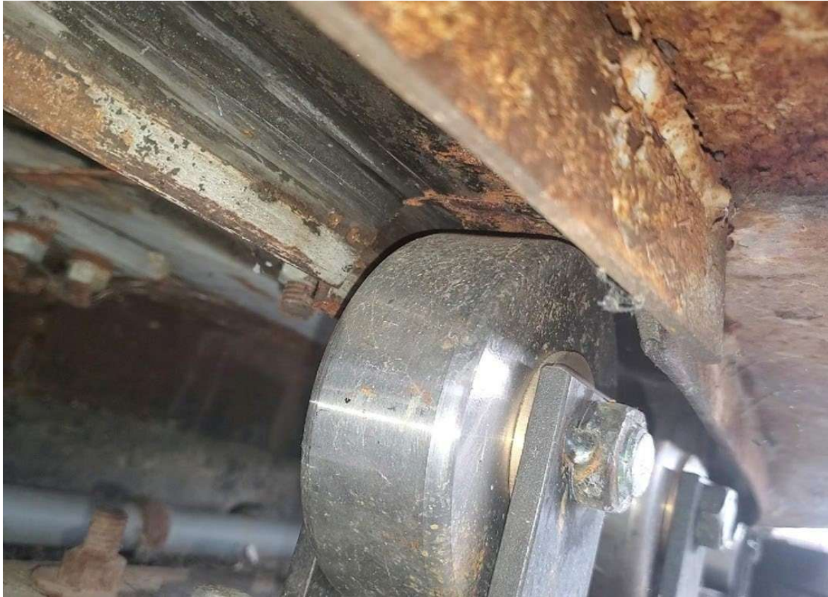
Bruneau Dunes Rail Deterioration at Old Observatory
