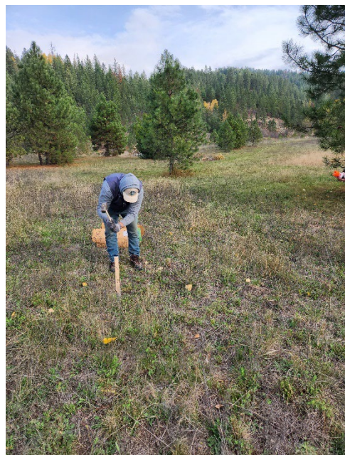
TCDA Park Manager Will Niska driving stakes in the ground for the centerline of the new campground road.
