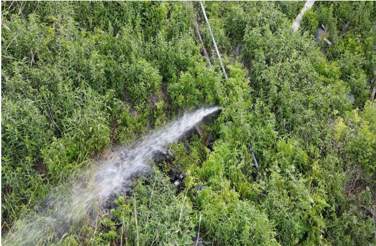
Irrigation Line Break at Ritter Island
