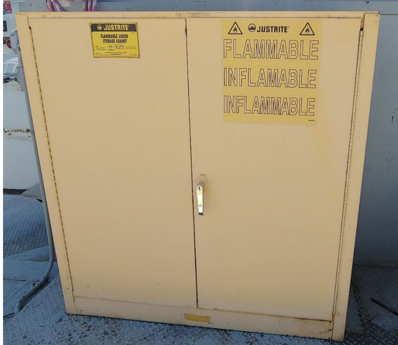
Figure 15-3. Locked flammables storage locker near floating fueling station at the Big Eddy Marina
