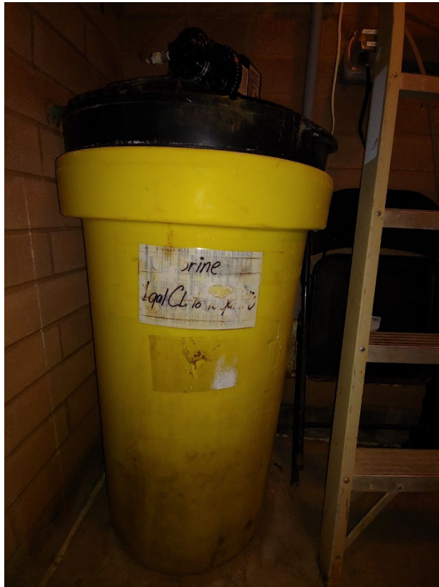
Figure 15-10. Poorly labeled 45-gallon chlorine tank at the Freeman Creek surface-water treatment facility
