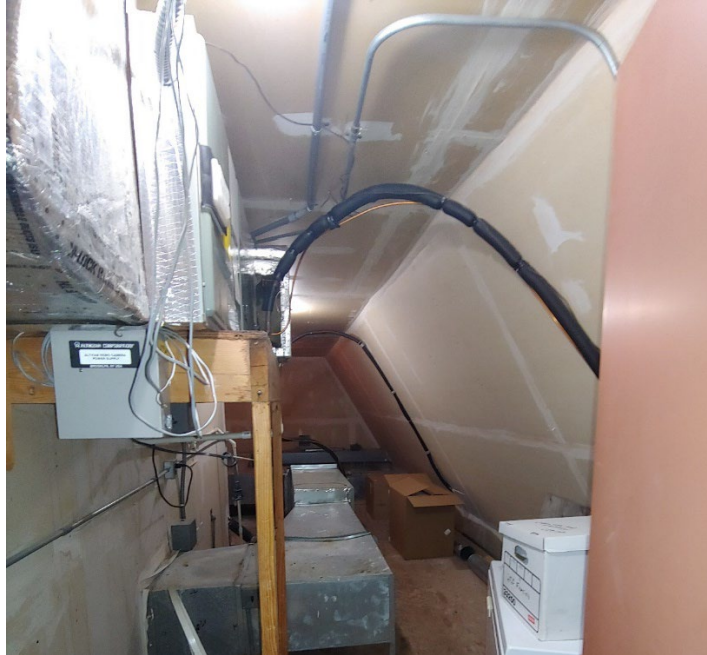
Figure 15-1. Heating and air conditioning equipment room in the Big Eddy Marina Lodge
