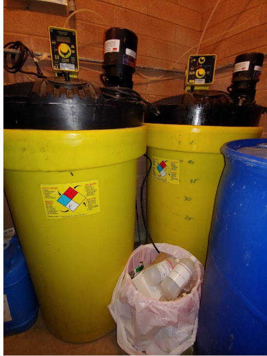
Figure 15-9. Two 45-gallon chlorine tanks in the Freeman Creek Campground surface-water treatment facility
