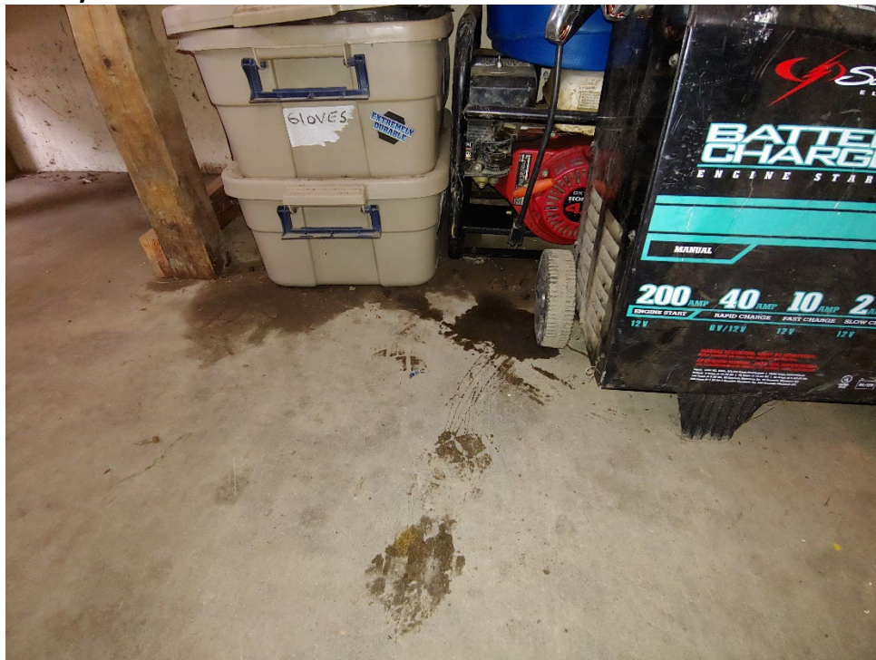
Figure 15-20. Stained floor near the generator in the Freeman Creek Campground maintenance garage
