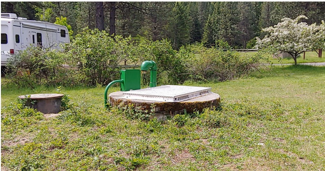
Figure 15-18. Freeman Creek Campground 3,000-gallon septic tank
