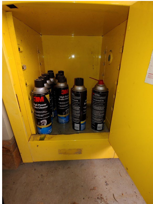
Figure 15-8. Flammables storage locker containing brake fluids in the Freeman Creek Campground Maintenance garage
