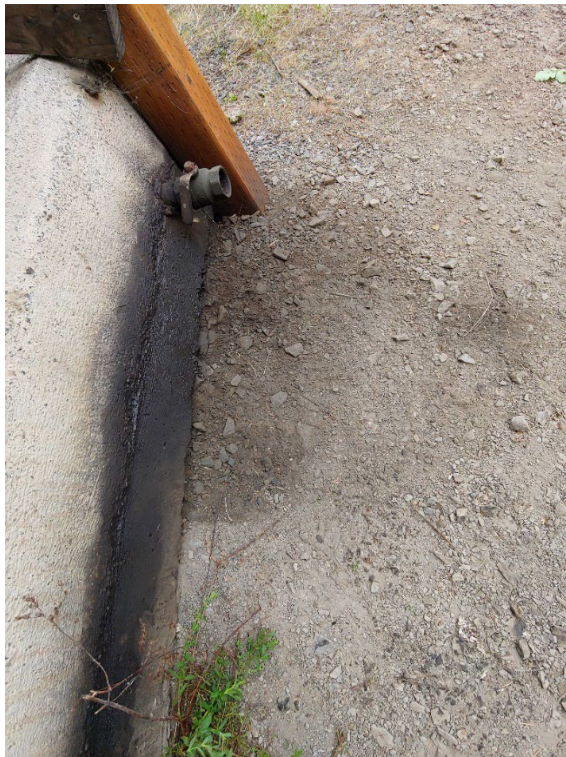
Figure 15-27. Stain soil and cement outside the 300-gallon diesel storage tank secondary containment at Freeman Creek Campground
