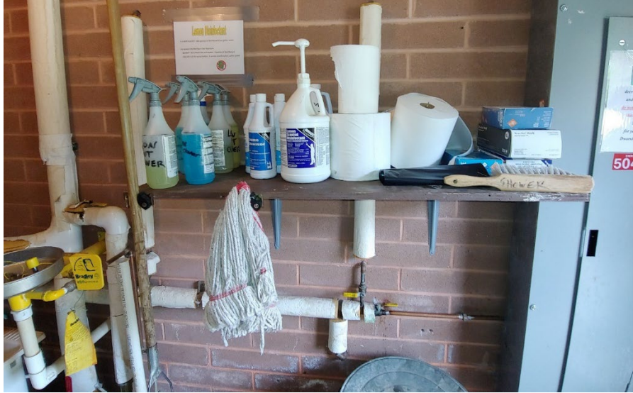
Figure 15-13. Bathroom closet with household chemicals at the Freeman Creek Campground maintenance garage
