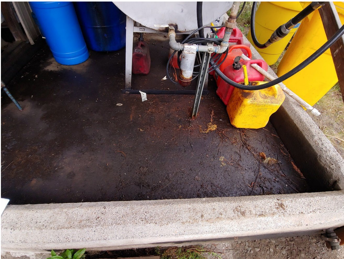
Figure 15-26. Stained cement floors of the 300-gallon diesel storage tank secondary containment at Freeman Creek Campground
