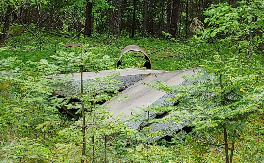
Figure 15-45. Discard concrete and metal culverts at Three Meadows Group Camp
