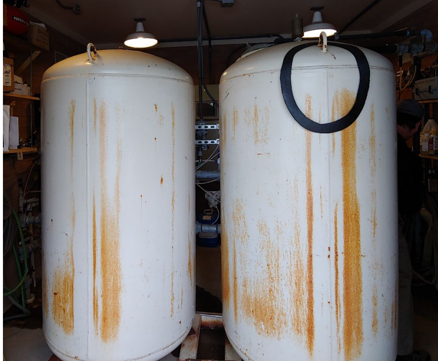
Figure 15-19. Water storage tanks in the Freeman Creek Campground surface water treatment facility
