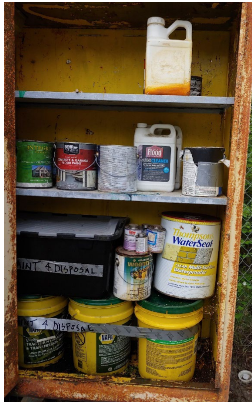
Figure 15-6. Content of a flammables storage locker at the Freeman Creek Campground maintenance area
