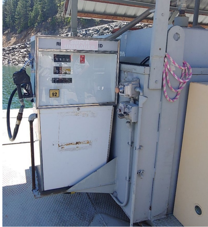
Figure 3-2. Big Eddy Marina On-The-Water Fueling Station
