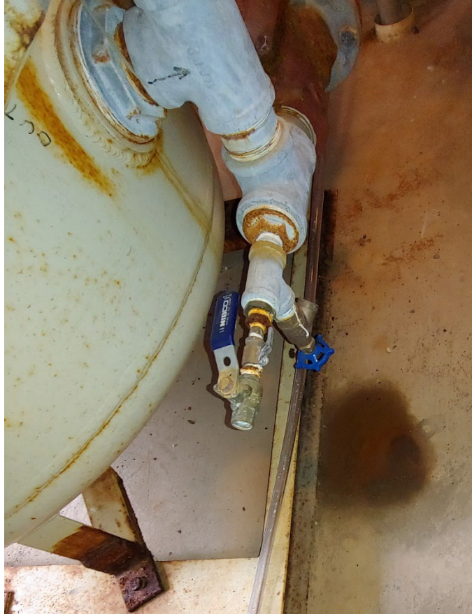
Figure 15-23. Staining on the cement floor underneath a water storage tank at the surface water treatment facility at Freeman Creek Campground
