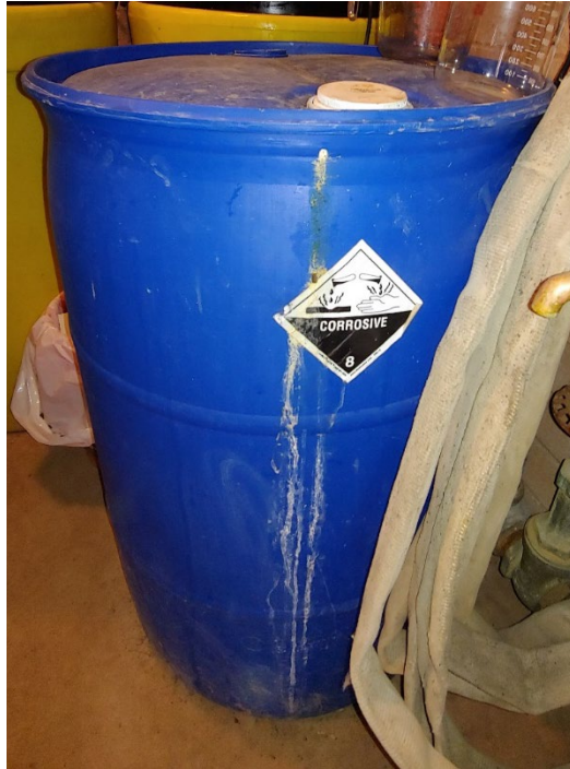
Figure 15-11. Unlabeled 45-gallon drum with corrosive sticker in the Freeman Creek Campground surface-water treatment facility
