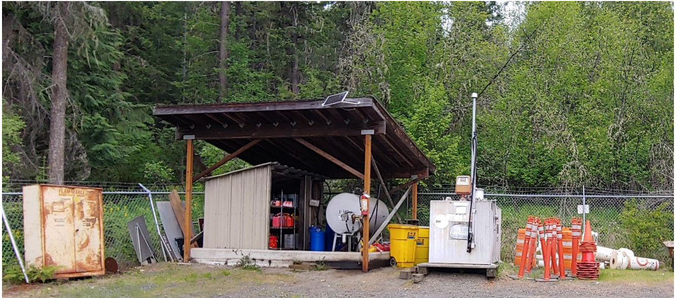
Figure 3-10. Freeman Creek Campground 300- and 500-Gallon Fuel Tanks
