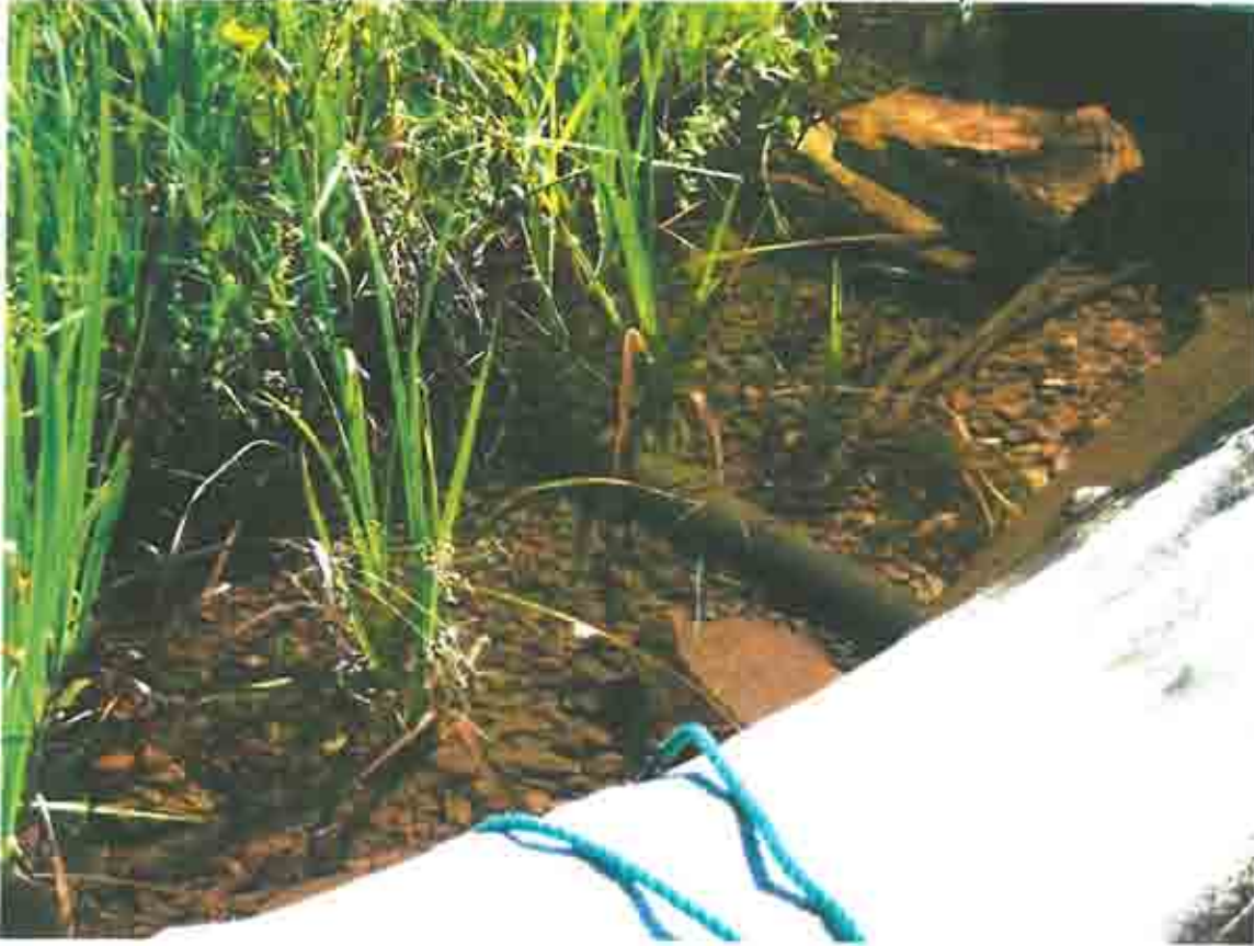
Fig 7. Sewer line going under ground at shoreline. This is the last you see of it.
