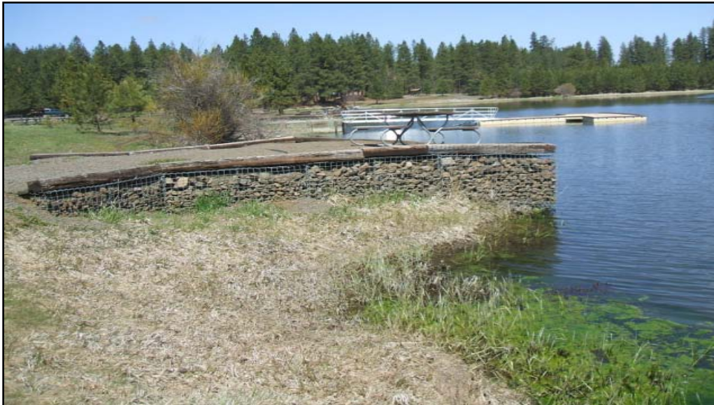
1.a Fishing Platform in Disrepair
