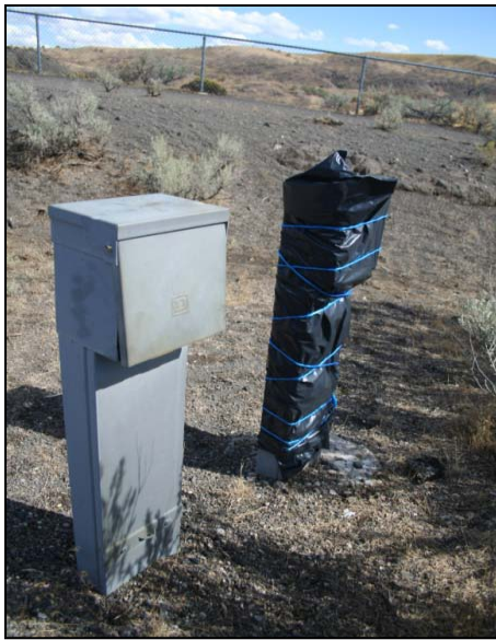
1.a Electrical Boxes in Disrepair
