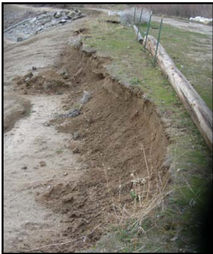
1.a Erosion of Shoreline
