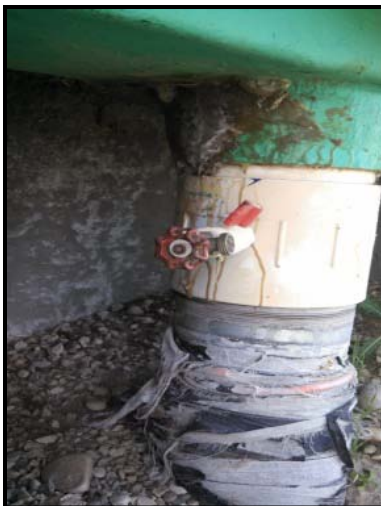
1.b Deteriorating Support
