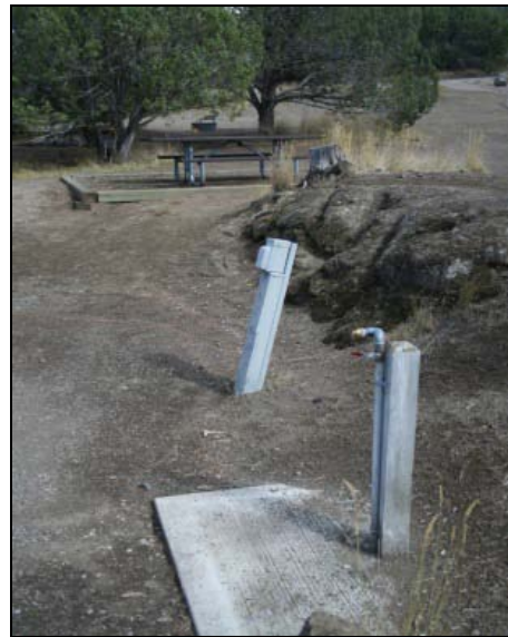
1.b Unstable Electrical Boxes
