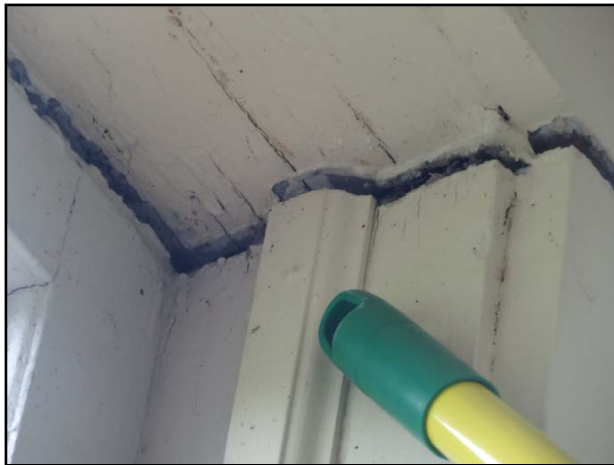
1. a Structural Failure
