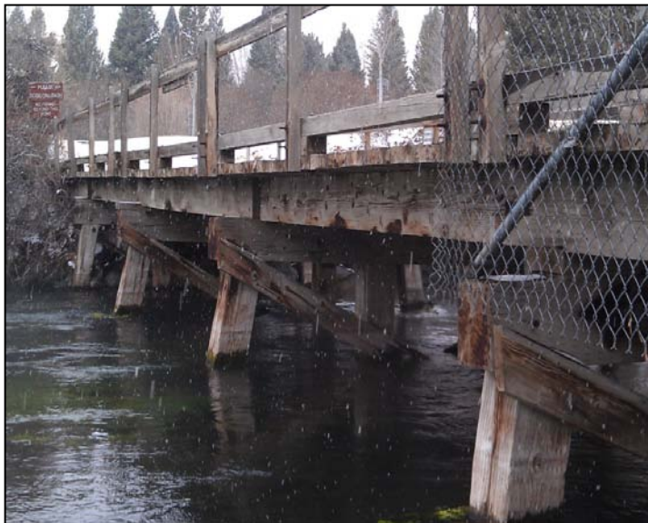
1.a Disrepair of Ritter Island Bridge
