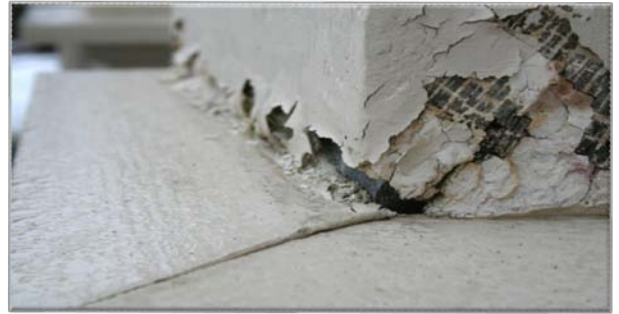
1.b Dry Rot at Base of Columns
