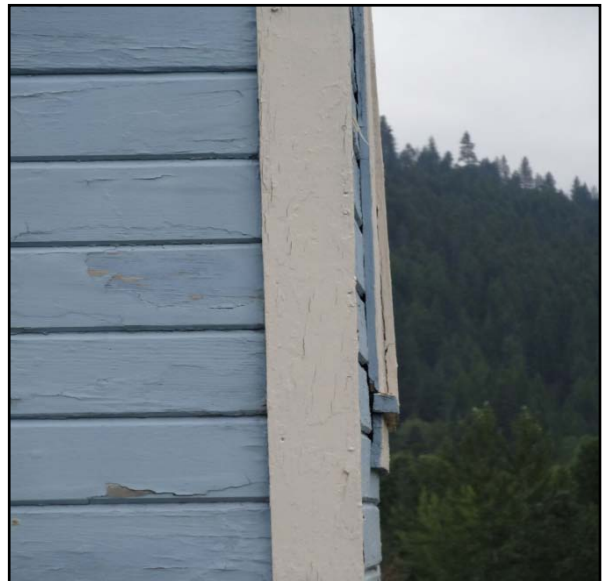
1.b Bowing of Wall
