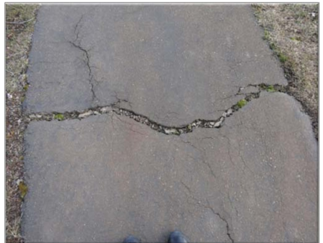
1.c Asphalt Trail with Numerous Cracks
