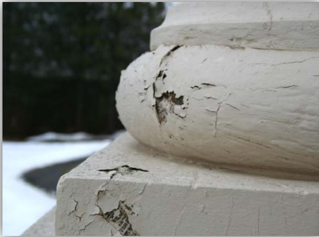
1.a Columns at Old Mission Church Dry Rot ( Repaired Several Times)
