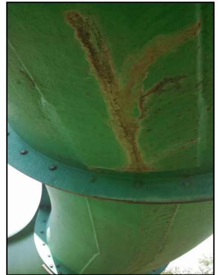
1.c Mended Crack in Water
