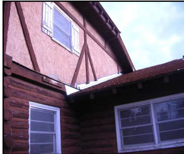
1.b Disrepair of siding and
