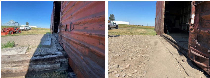
Entrance ramp to box car before and after.
