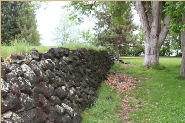
One of the rock walls built by the CCC at Lake Walcott State Park
