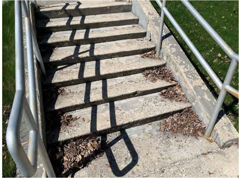
Concrete Stair Exhibiting Spalling
