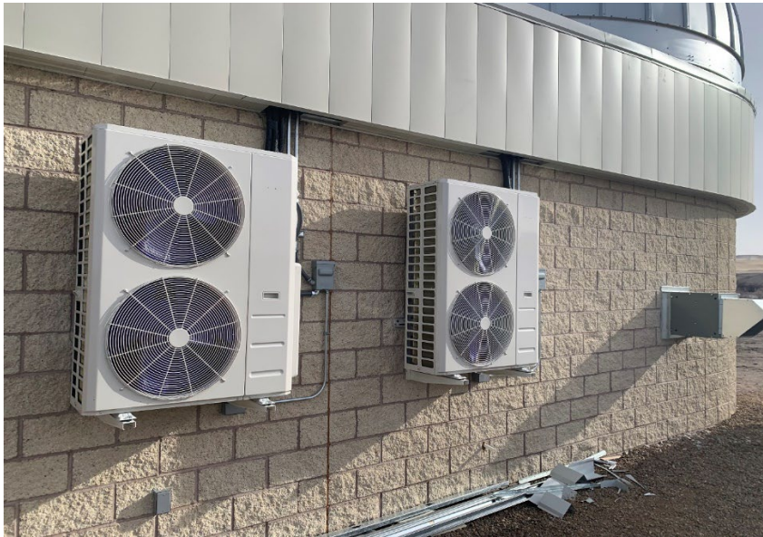
New Observatory HVAC
