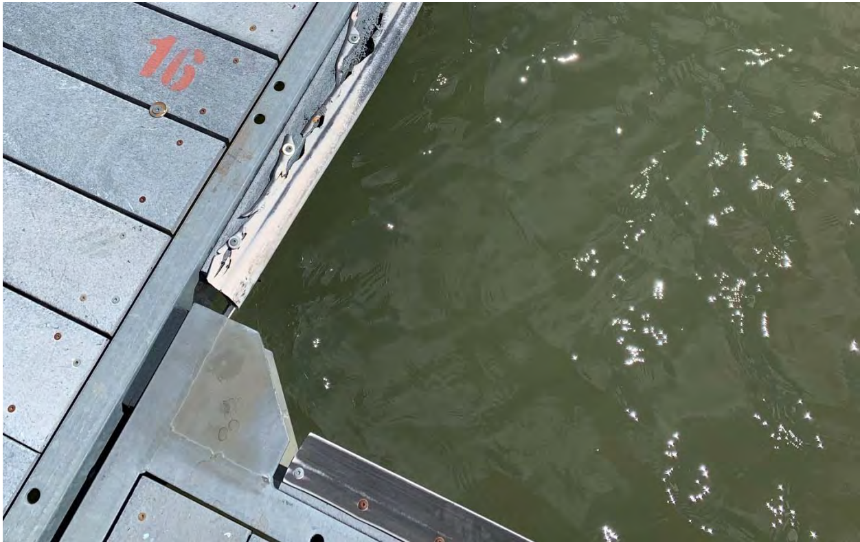
Typical Finger Pier Connection With Rubber Spacer and Needed Fender Replacement
