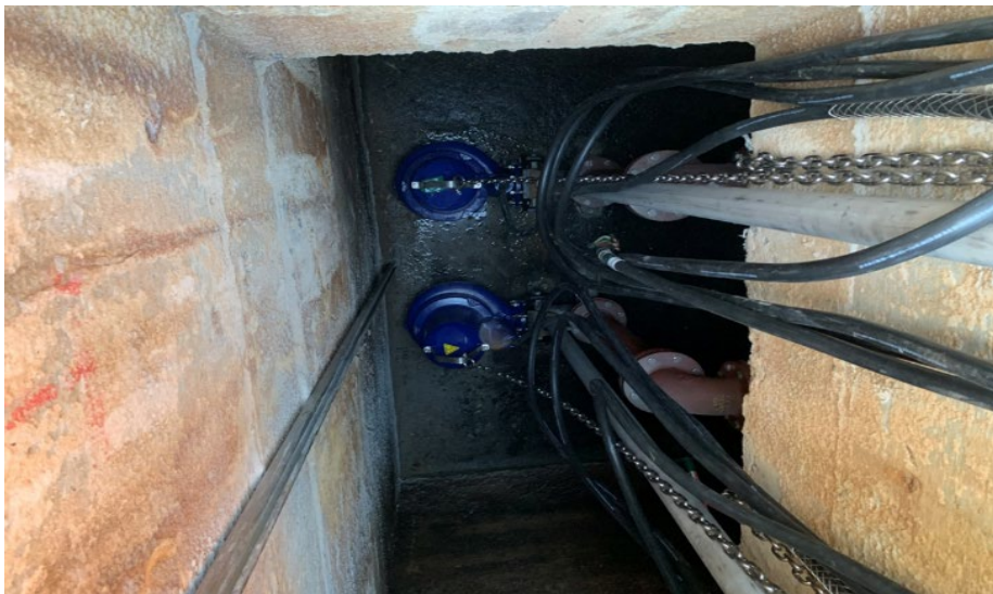
New lift station at Eagle Island
