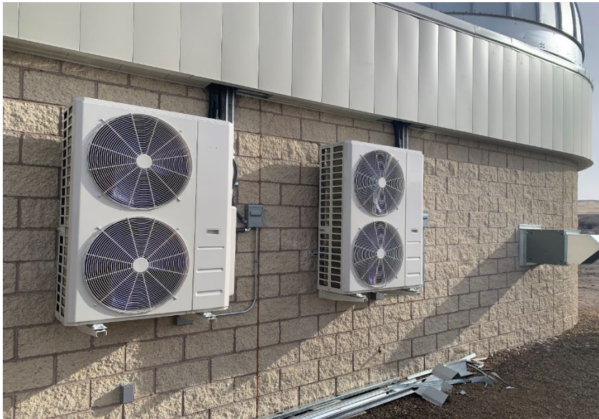
New Observatory HVAC
